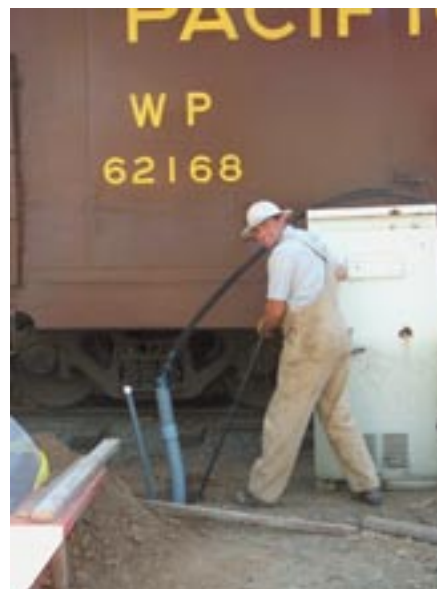
Lee Frechette on one of many his work days installing the new power conduits and wires.
