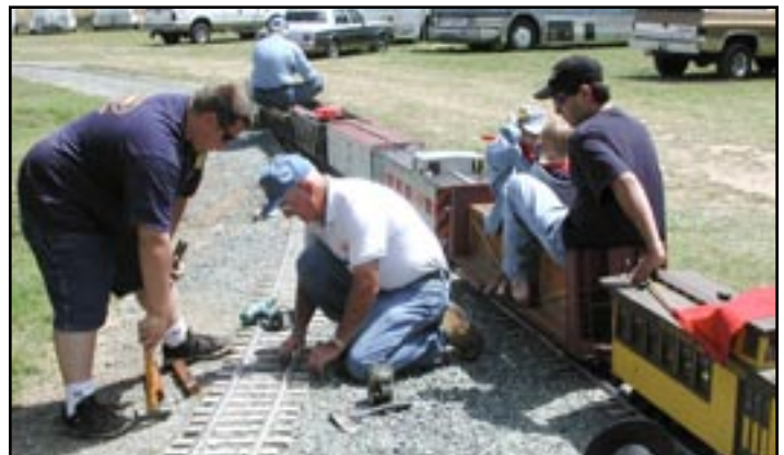
Track repair crew Richard Lutrel and Pete Arney adjusting rail to reduce caps at the rail joints during the Spring Meet.
