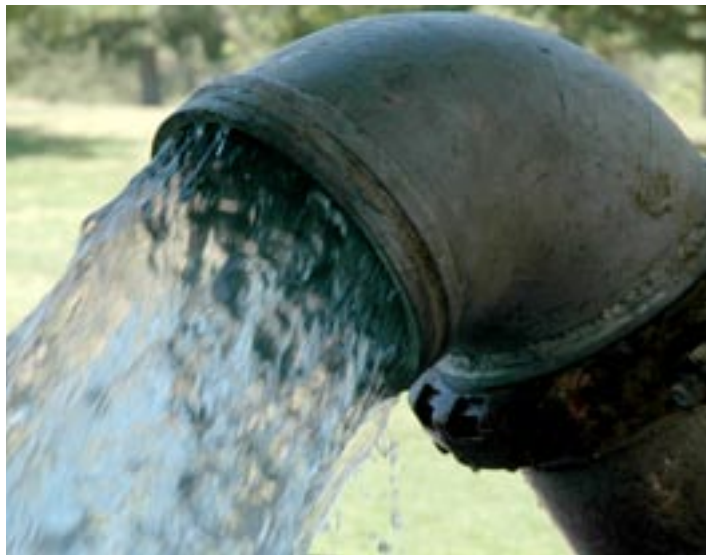
The new well that was being drilled over the last several weeks for the Hagan Park seems to have found the water it wanted. They were testing it on June 21st and it was pumping over 900 GPM = that is 900 gallons per minute in the 10 inch pipe. Too bad its not oil we could all be rich. Anyway this will give the park a much better supply of water to keep things green during the summer months.
