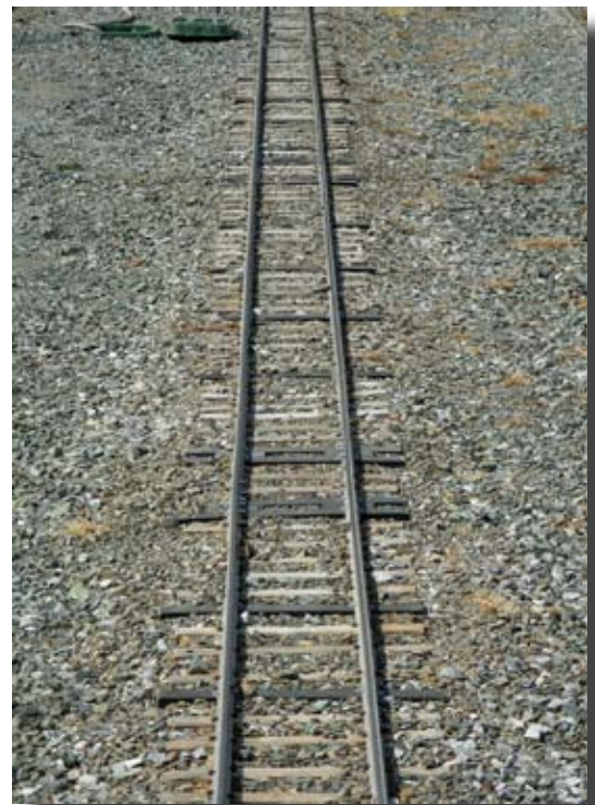
Ongoing tie replacement on main line continues with replacing every 5th tie with a plastic tie and new long splice bars with extra tie support under each joint.
