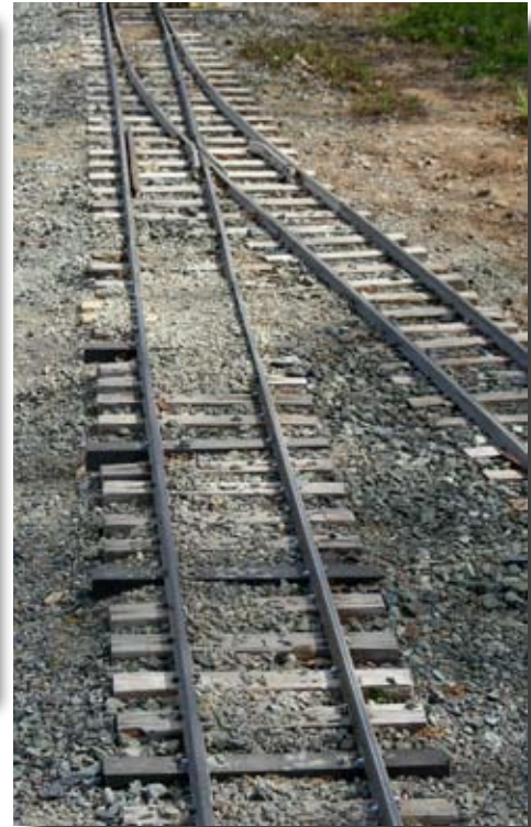
The switch at Hill View West has a new smother ride and sound. The multi-spliced rail has been replaced. Now instead of many joints inches apart there are two joints 12 feet apart.
