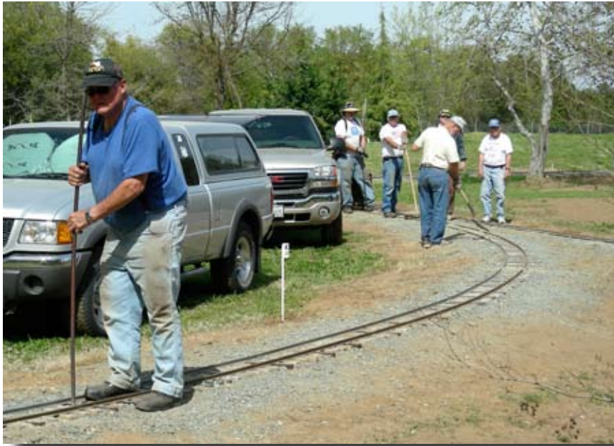
Darrell and his track crew has been very busy the last few weeks. Here they have replaced 88 feet of Aluminum rail with steel rail along North Curve. Replacing some ties and adding ballast.
