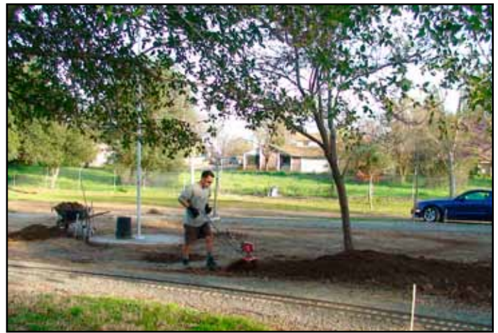
Andy is busy working on landscape for the new memorial. The Granite memorial will be in place with a dedication in May.
