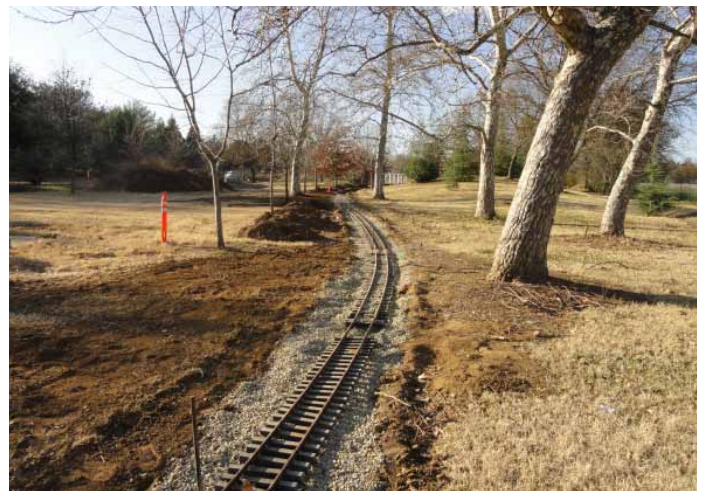
Mainline looking toward north - waiting for final alignment and ballast - where is a tractor when you need one.
