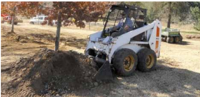
Chris Johnson of CJC Contractors in Rancho Cordova who heard of our stolen tractor volunteered with his Bobcat tractor and made quick work moving our piles of dirt - Thanks Chris
