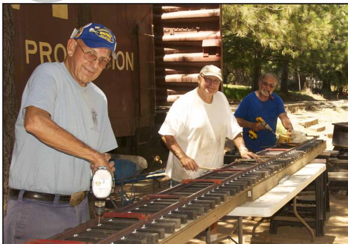
Tom, Paul, & Scott building track panel. It is great to have such hard workers.
