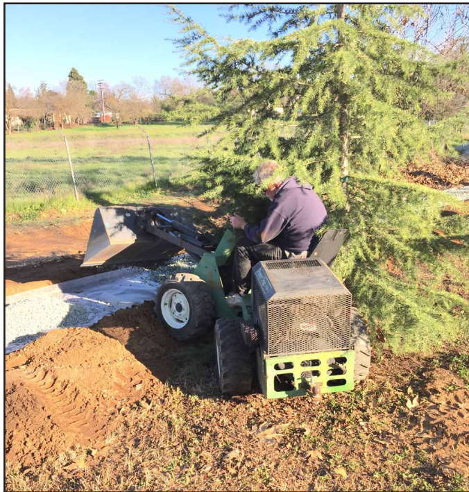
Steve Perry making the extra effort moving ballast to the correct spot along the new graded right-of-way for Twin Bridges.
