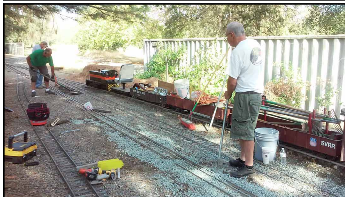
Replacing ties in the upper yard coming out of the steaming bays.
