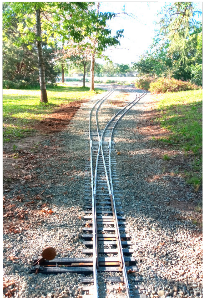
New switch to select Main Line to Hill View or new passing siding and to new tank farm sidings.
